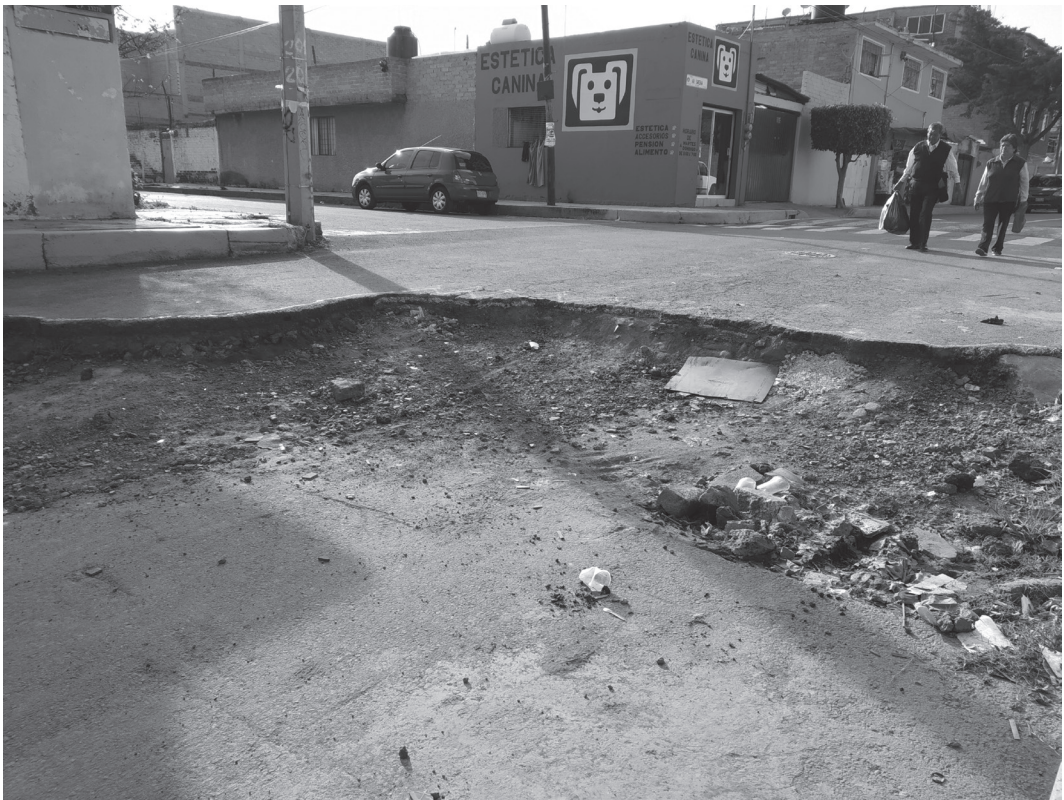
Fig. 1 – Cracked street 18 months after the earthquake (photo Luis Razzo).
